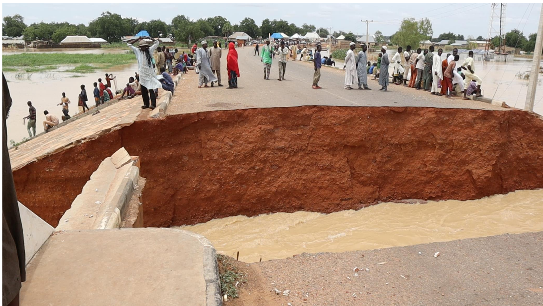
Bridge washed away by flood in kebbi state
